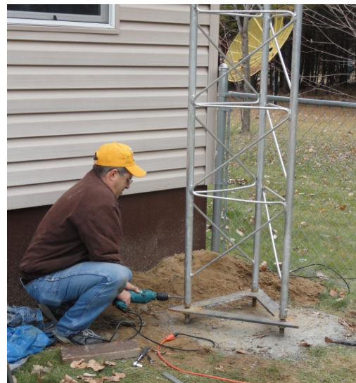
Bottom right shows KDØERE drilling a hole to secure the mounting of the base of the tower. Photos here are not in chronological order.
