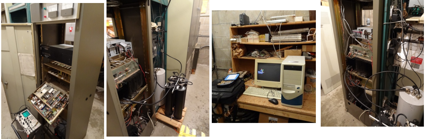
Photo of the installation with test equipment. Pix and write-up provided by Roger WØWUG.
